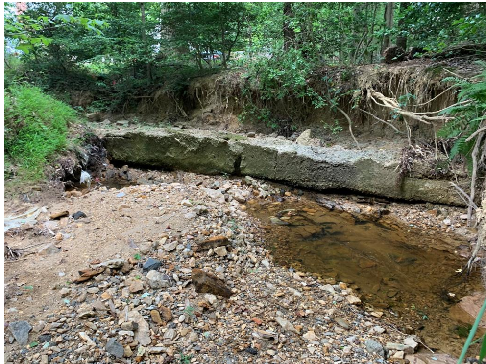
Eroded channel and exposed sewer line at Trapp Rd outfall.
